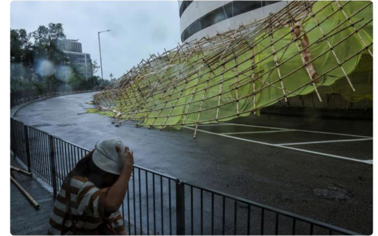
Collapsed bamboo scaffolds of a residential building are seen as Typhoon Wipha approaches, in Hong Kong, China, July 20, 2025. REUTERS/Tyrone Siu © Thomson Reuters
